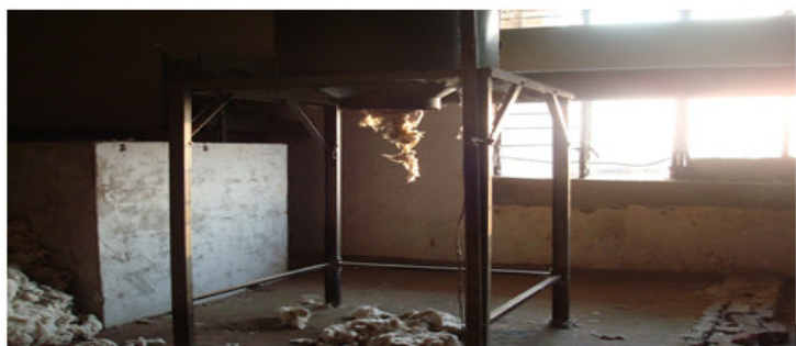
Figure 3 Cotton Waste – Waste Room
